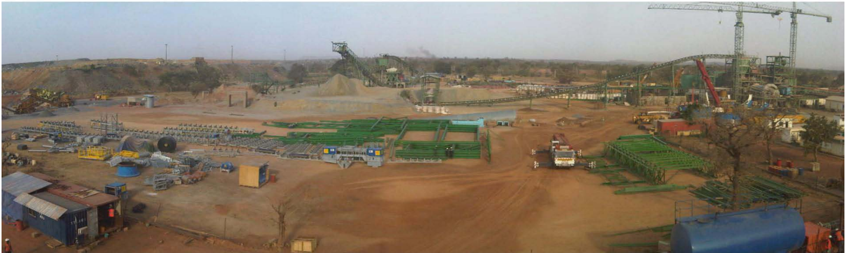
Milling Facility – expanding to 4,000 tpd
